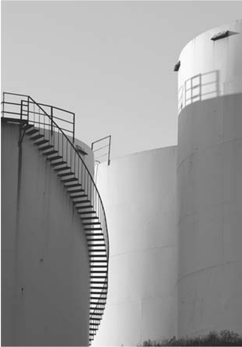
FIGURE 3.4 Outside aboveground storage tanks
