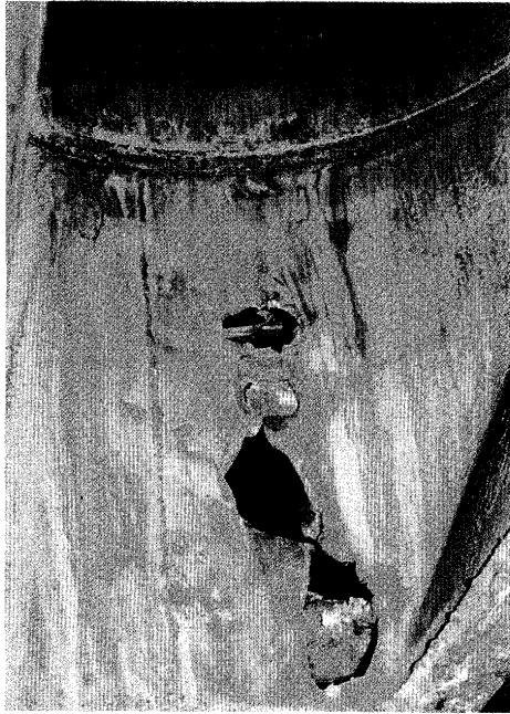
The exhaust gas pipe was holed by the pieces of the T/C casing of the M/E blown off by an explosion.
